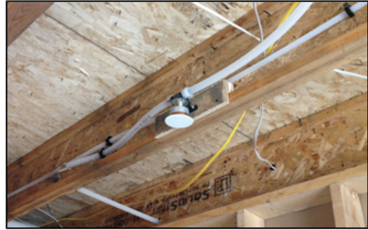
All Eco Village homes feature Uponor crosslinked polyethylene (PEX-a) plumbing and multipurpose fire sprinklers throughout, with radiant floor heating in the homes with basements.
