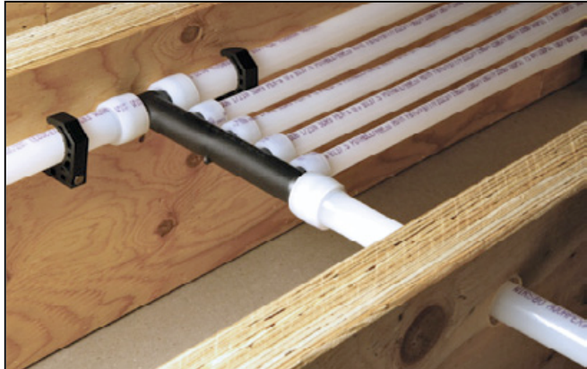
EIR: The adoption of PEX tubing into the California Plumbing Code would be “an environmentally superior action with respect to public health and hazards, water quality and air quality.”
