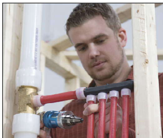
Building Standards Commission approves PEX for water distribution: a victory for the trade and for the consumer in California.
